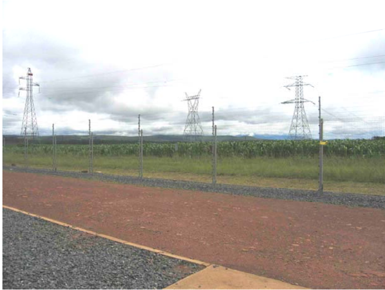
Photo 2: Photograph of Eros substation showing maize fields on the site of the proposed extension.
