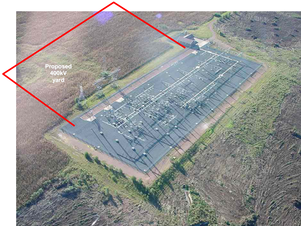
Photo 1: Aerial photograph of Eros substation showing receiving environment and extent of proposed upgrade
