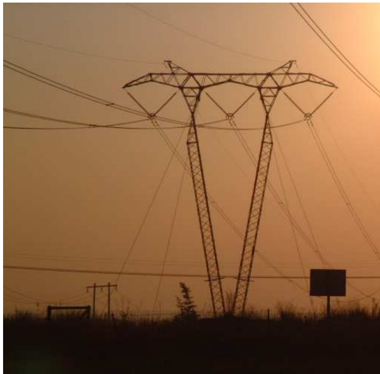
Figure 31: Guyed suspension tower
