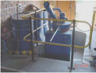
Typical crushing plant
