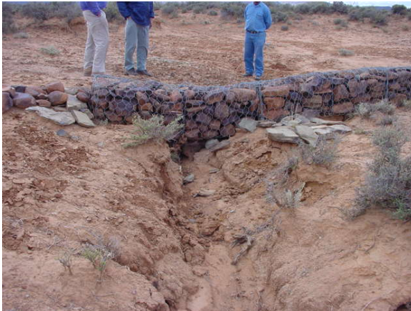
Figure 5. An example of an inappropriately designed gabion. No geotextile or apron was used in this case and erosion eventually occurred under the structure. No provision was made to prevent erosion at the overflow.
