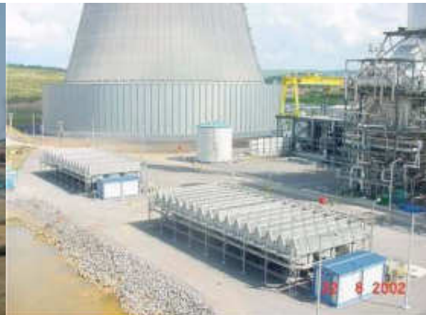
Figure 4.5 Photograph showing a power station with the water-to-air heat exchangers of the Stack-in-Tower system of indirect dry cooling technology
