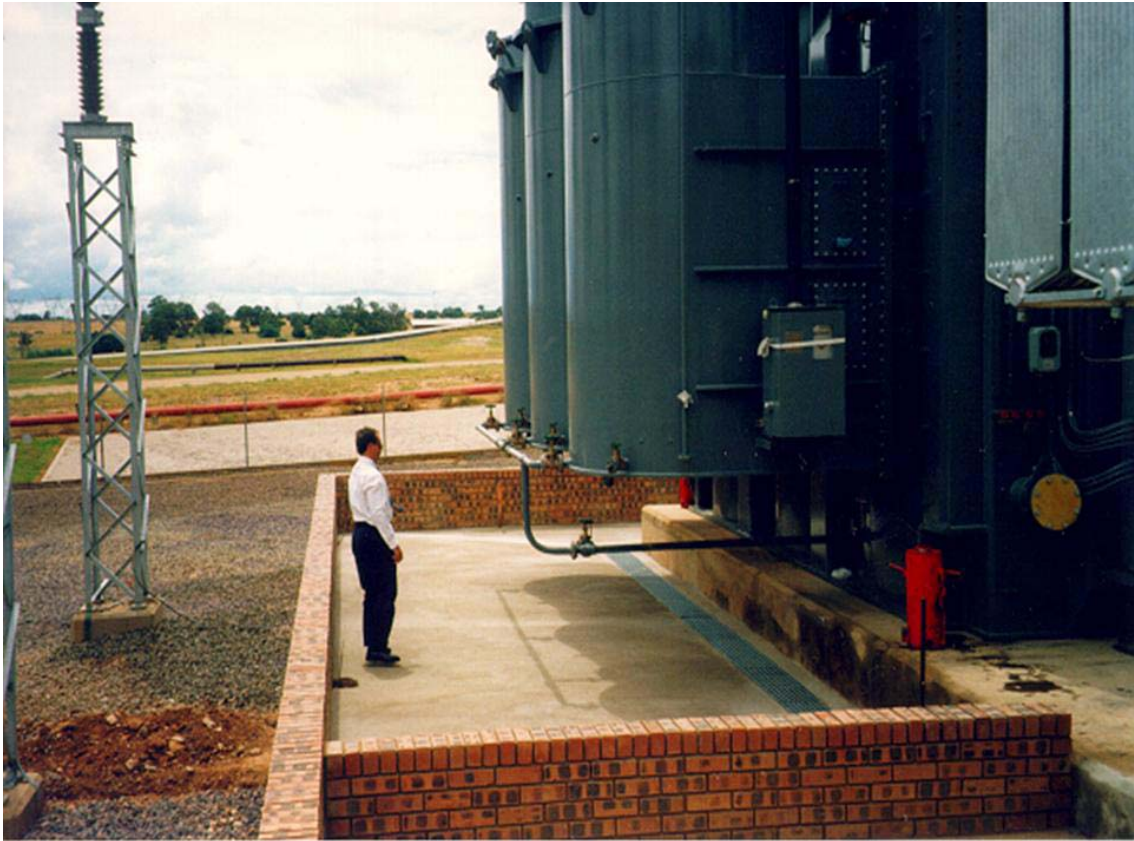
Figure 7 Transformer and bund wall
