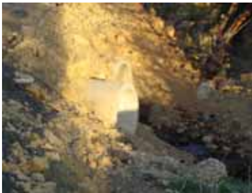
Plate 7: Inadequate storm water management structures
