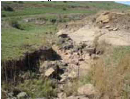
Plate 5: Erosion gullies associated with poor stormwater management
