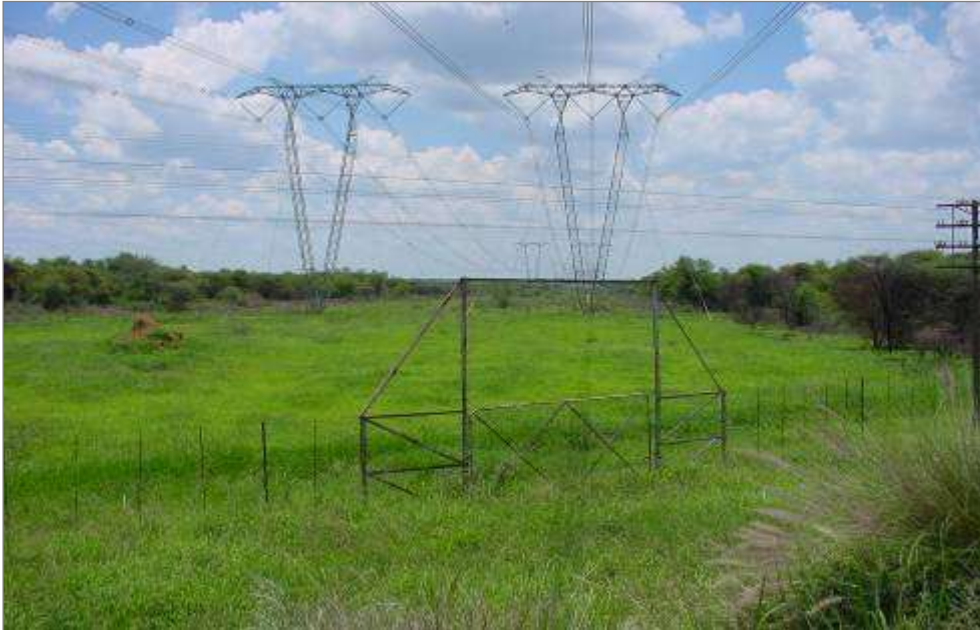
Figure 35: Access gate for an Eskom transmission line
