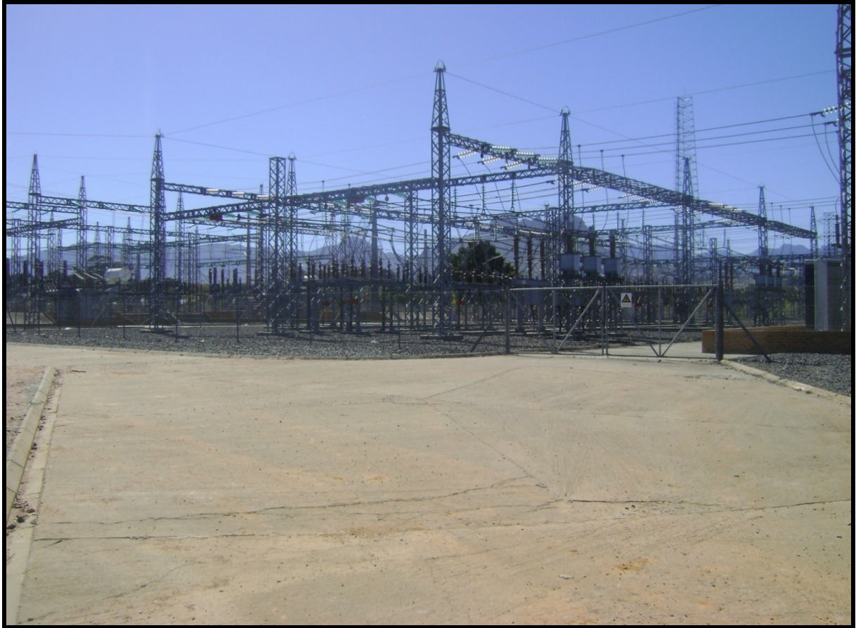
Figure 2: Firgrove MTS substation entrance
