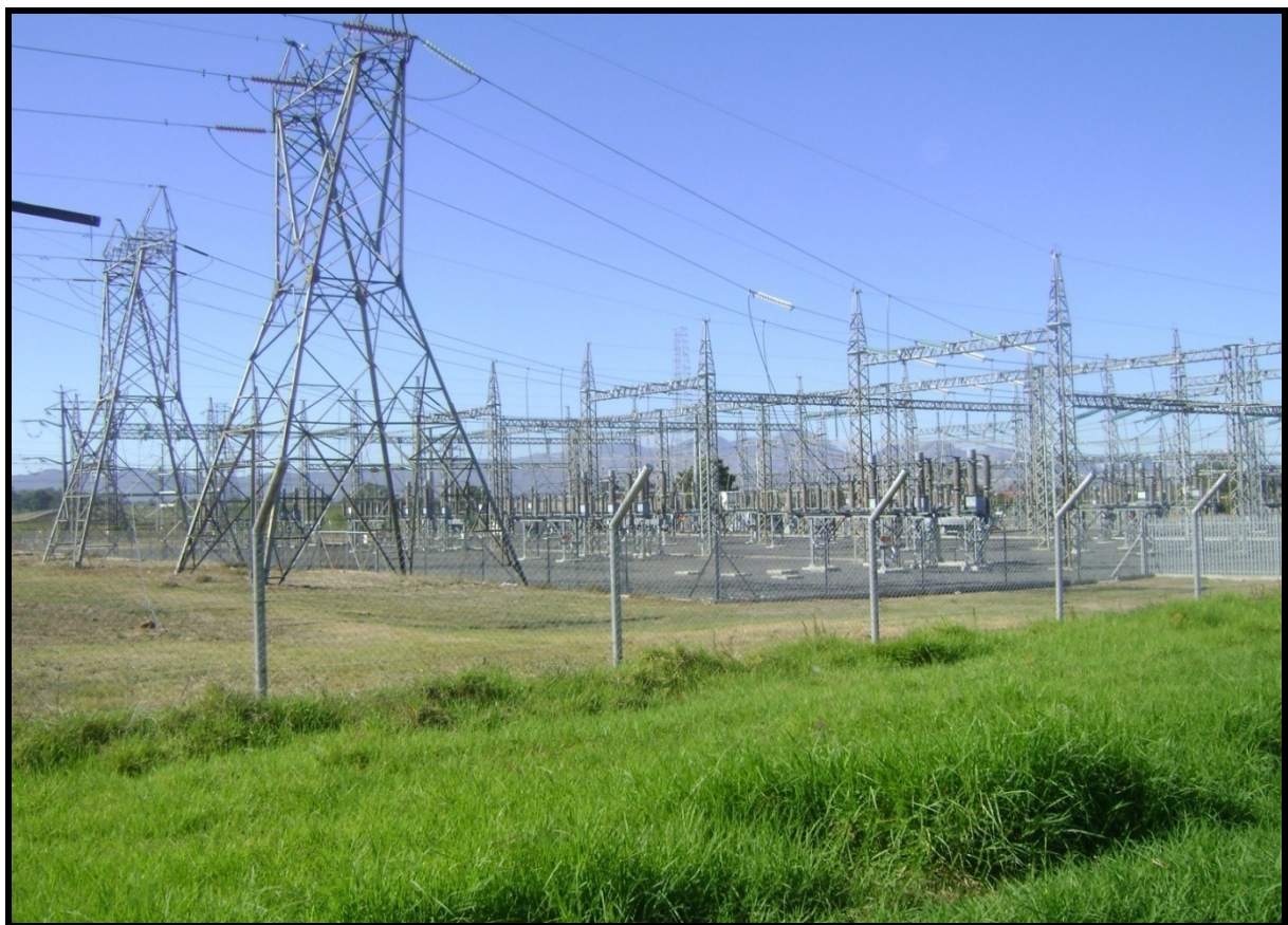
Figure 1: Firgrove MTS substation
