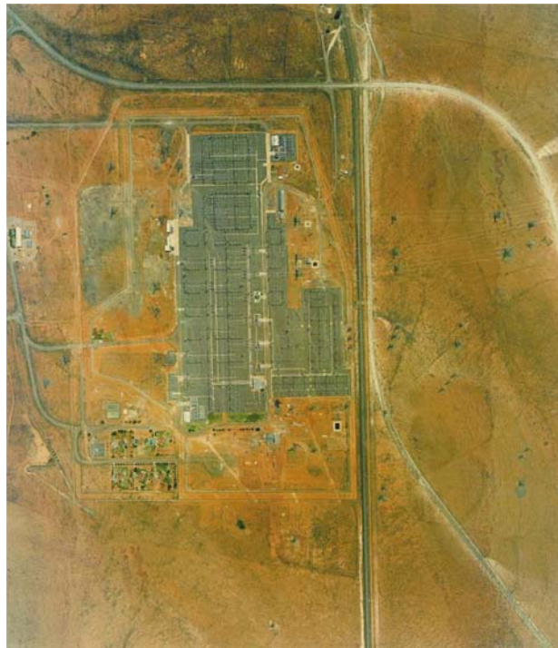
Figure 7 Hydra Sub-station that is typical of Eskom Sub-stations in South Africa
