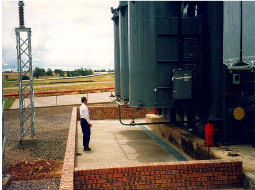
Figure 8 Transformer and bund wall
