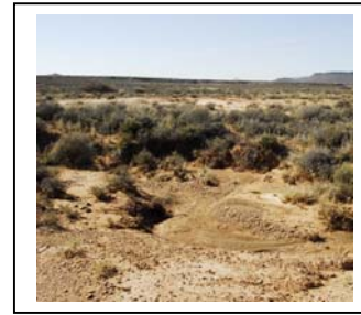
A165 Erosion prone area
