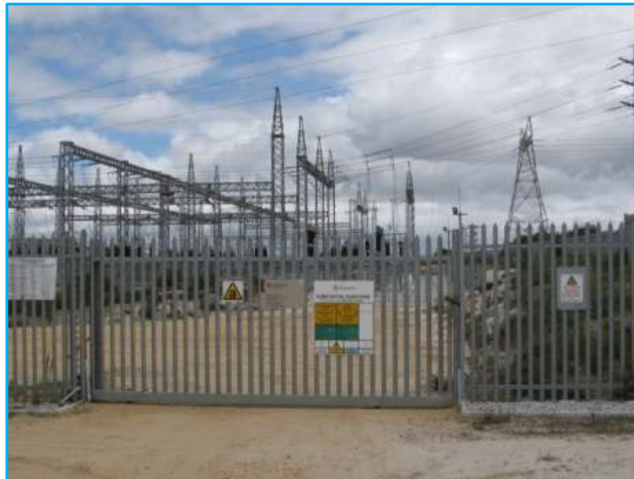
Existing Houhoek Distribution Substation
