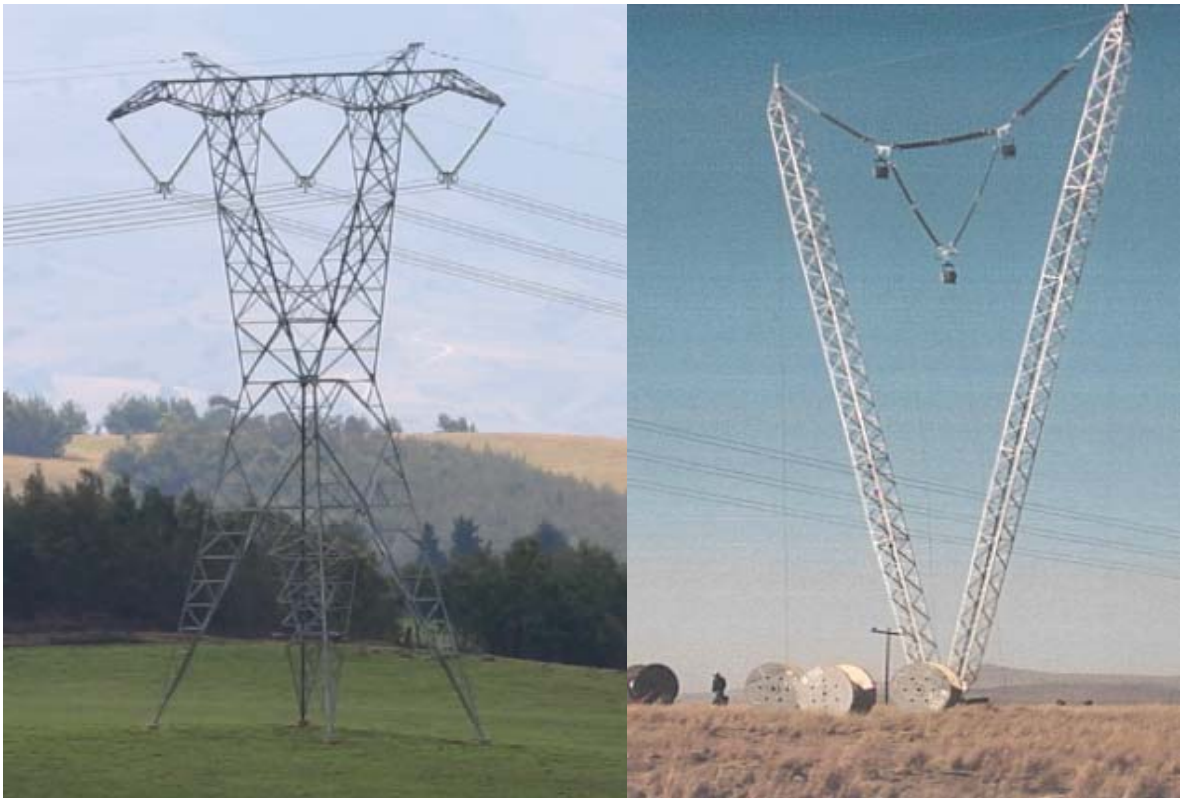
Figure 2c: Examples of both strain tower and compact cross rope suspension tower types
