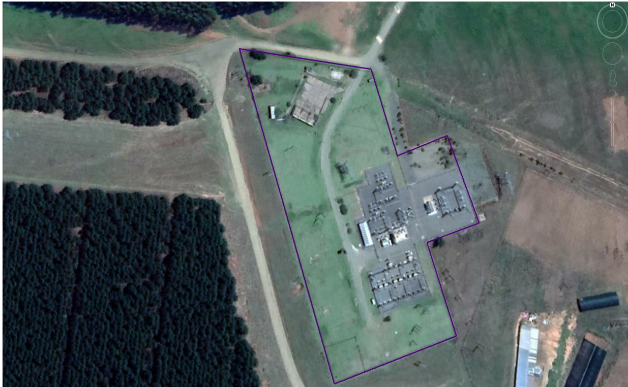
Figure 6: Aerial Snapshot of the Existing Elandskop 88kV Distribution Substation (Google Earth Image, 2018)
