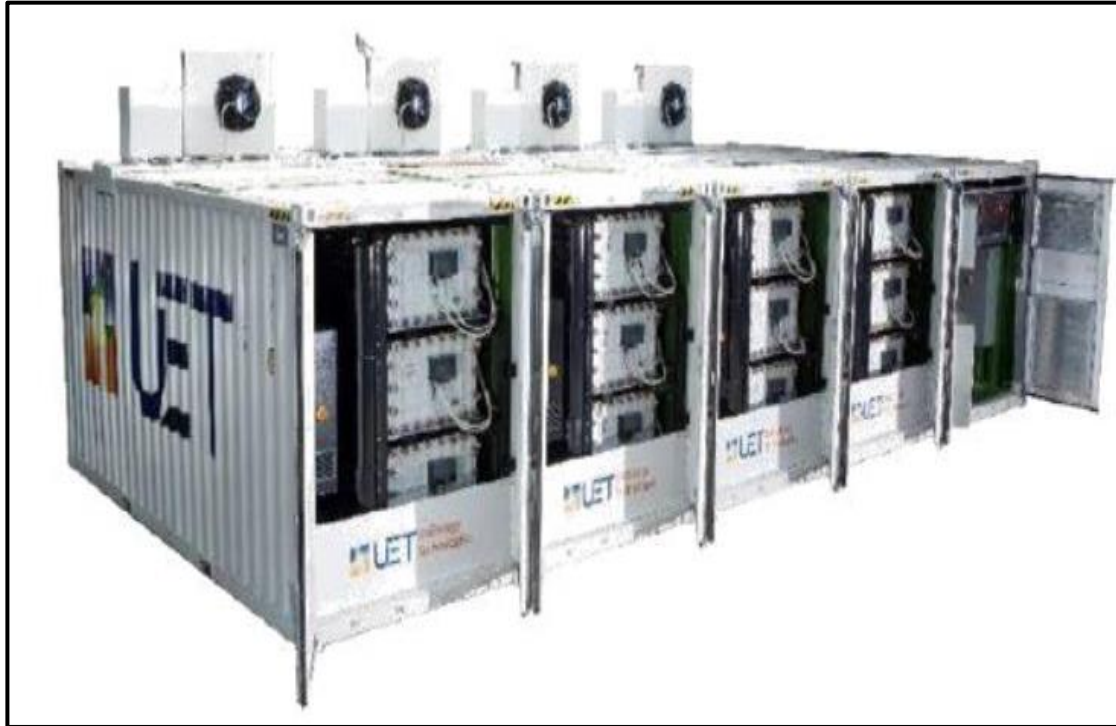
Figure 9: Flow Batteries – Vanadium Redox Battery
