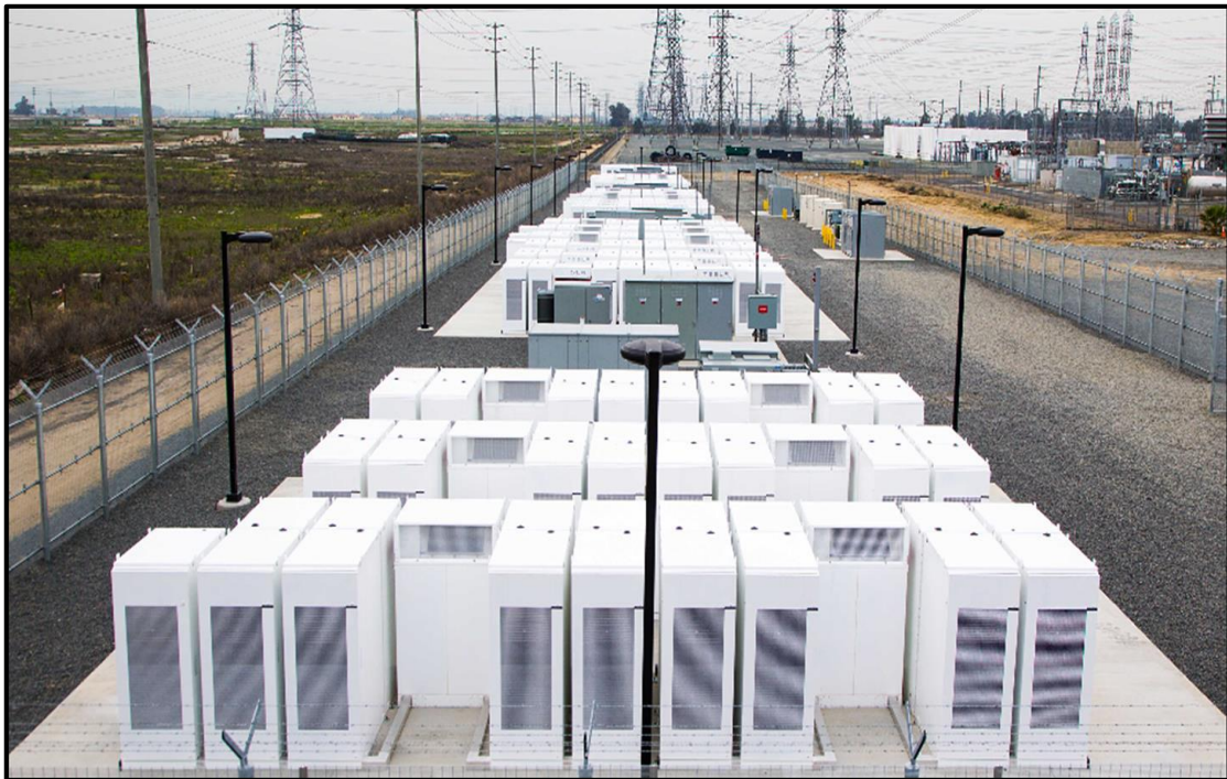
Figure 8: Solid State Batteries
