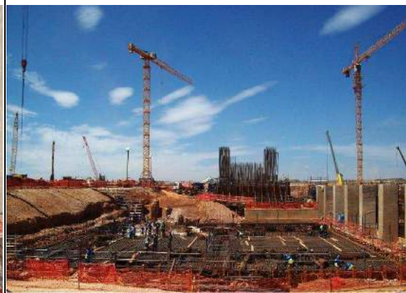
Turbine Generator Area - Unit 1 January 2010
