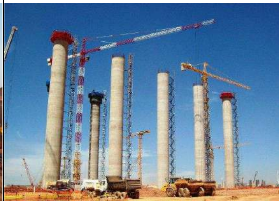
Air cooled condenser columns - Unit 1 January 2010
