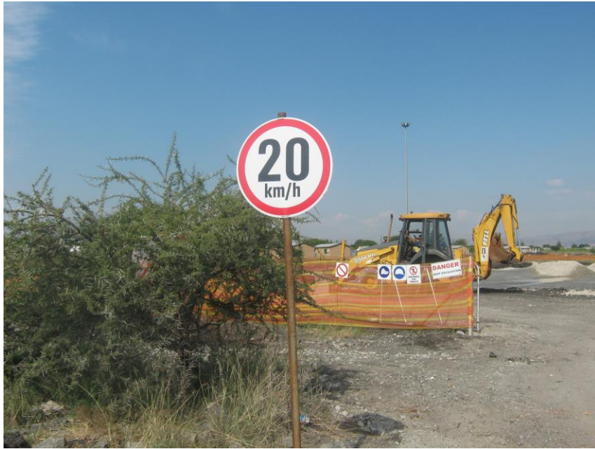
Photo 8: Safety warning signage in place.
