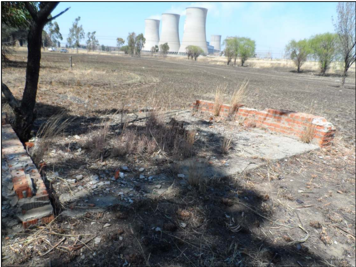
Figure 14 - Red clay brick and cement ruin
