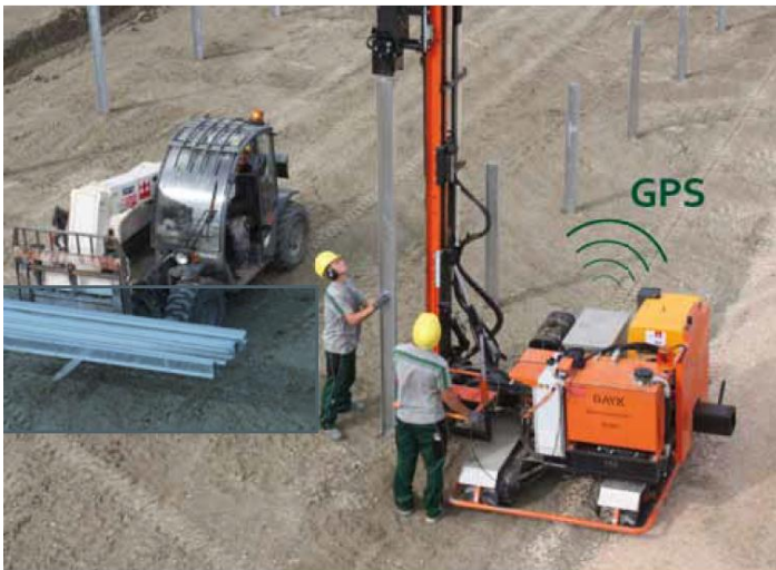
Figure 3: Typical machine used to drive or ram the piles into the ground
