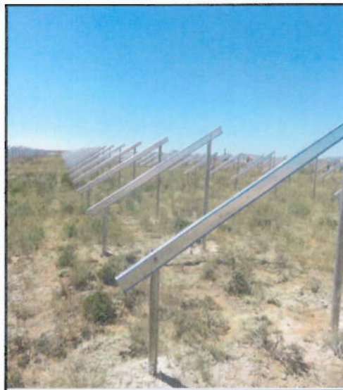
Figure 1 A typical PV array - The PV panels are attached to the mounting structures, that are then inserted into the ground (either rammed, screwed, etc).
