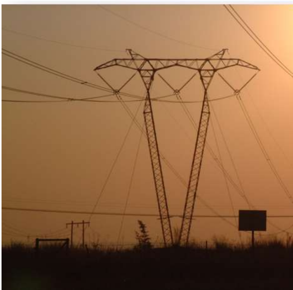
Plate 4: Guyed Vee Tower
