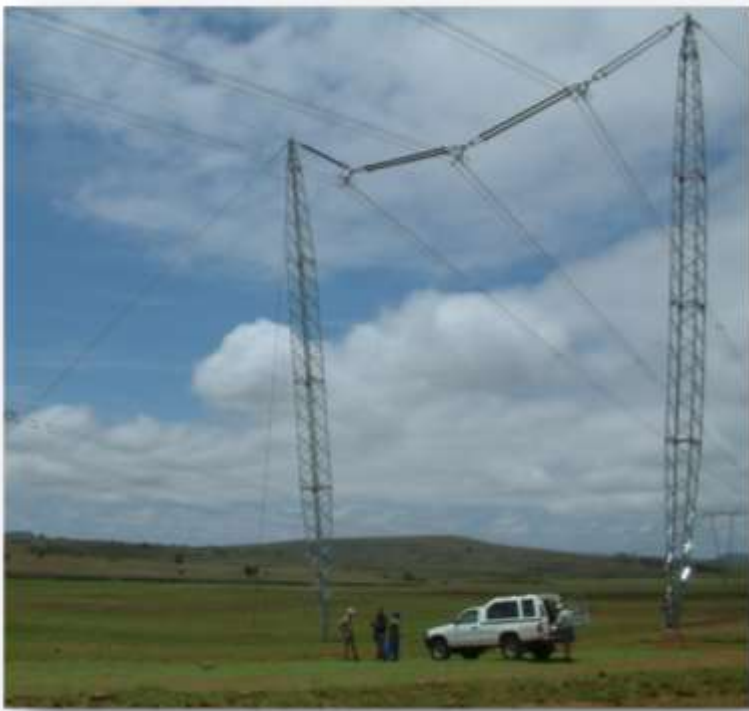
Plate 2: Cross Rope Tower
