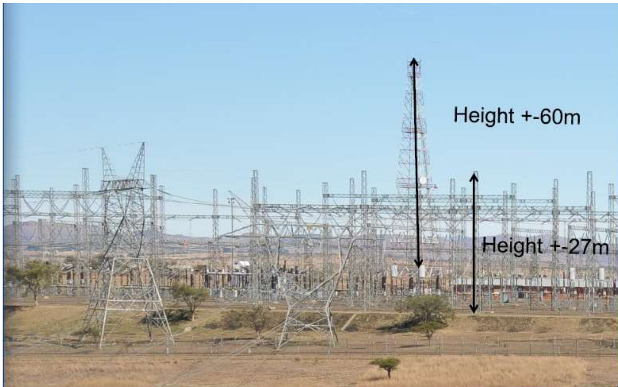
Figure 3.2: Side view of typical substation site
