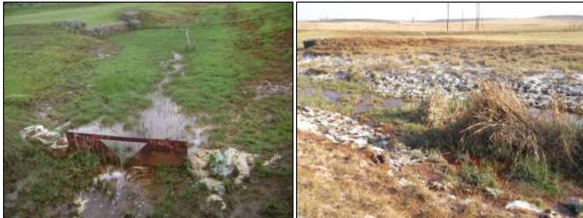
Figure 5-8: Decant emanating southeast of the Discard Dump
