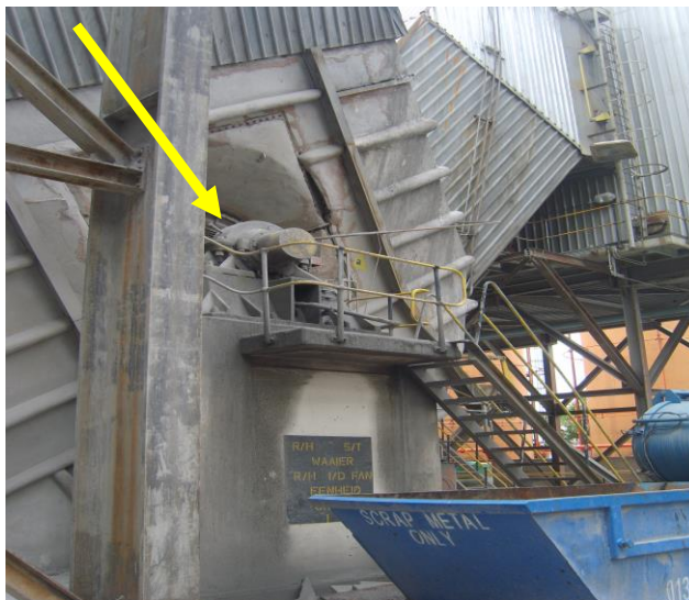
Figure 6: ID Fans to be upgraded at Kriel Power Station
