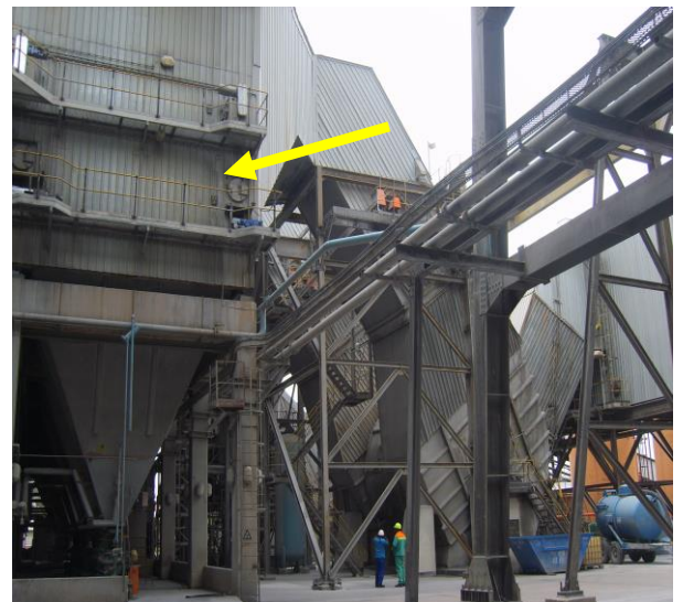
Figure 7: Existing Electrostatic Precipitators at Kriel Power Station
