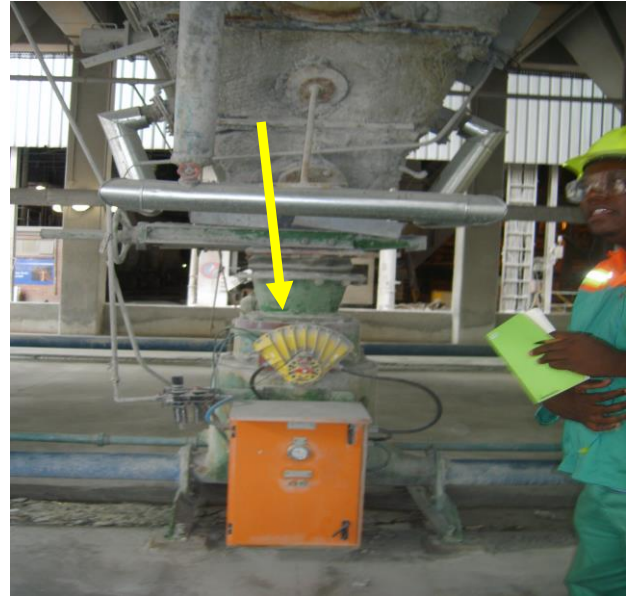
Figure 5: Pressure Vessel situated under the footprint of the FFP casing
