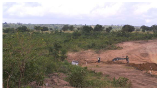
Figure 80: Construction having a negative impact on natural vegetation and streams – erosion severe.
