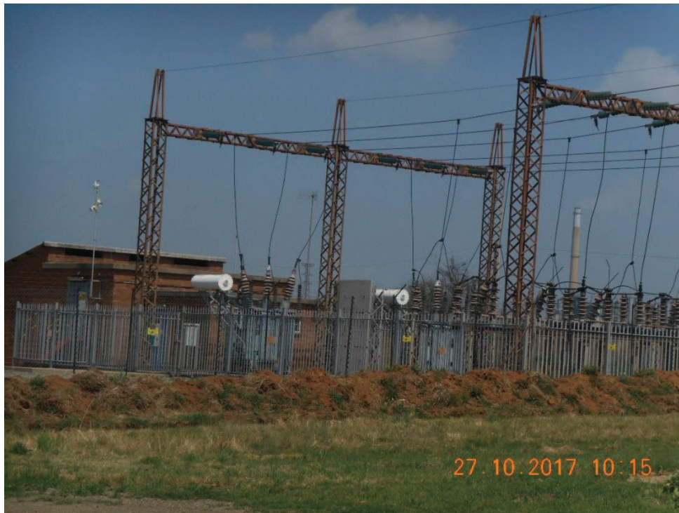
Figure 7: Photograph of the Mookodi substation
