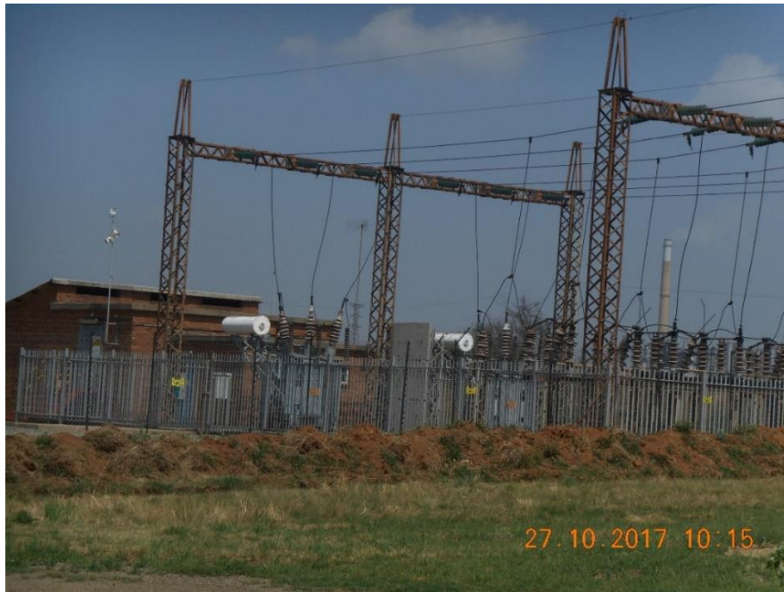
Figure 7: Photograph of the Mookodi substation
