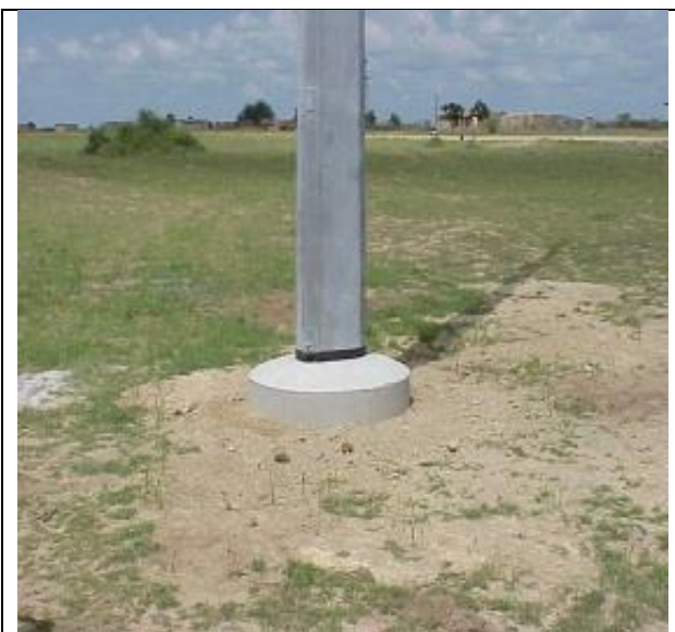
Figure 1-3: Single circuit steel mono-pole structures to be used for the Pylon structures
