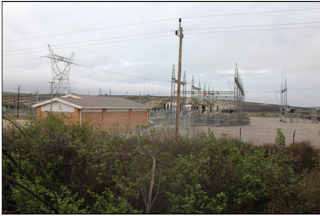
Figure 3: The Paleisheuwel Substation
