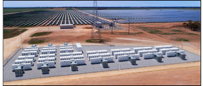
Figure 5: Example of a BESS
