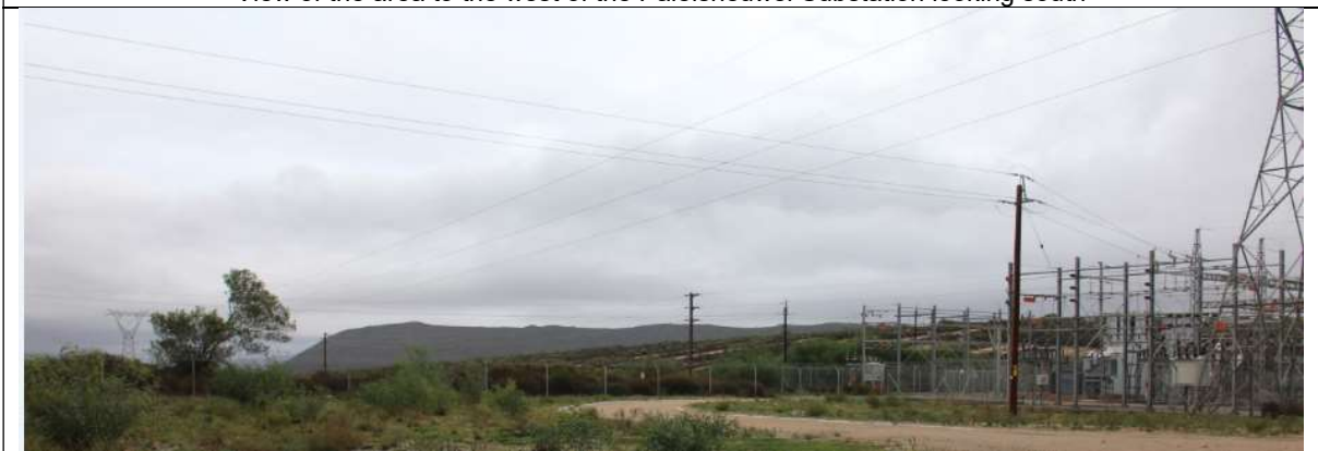
View of the Paleisheuvel Substation looking south
