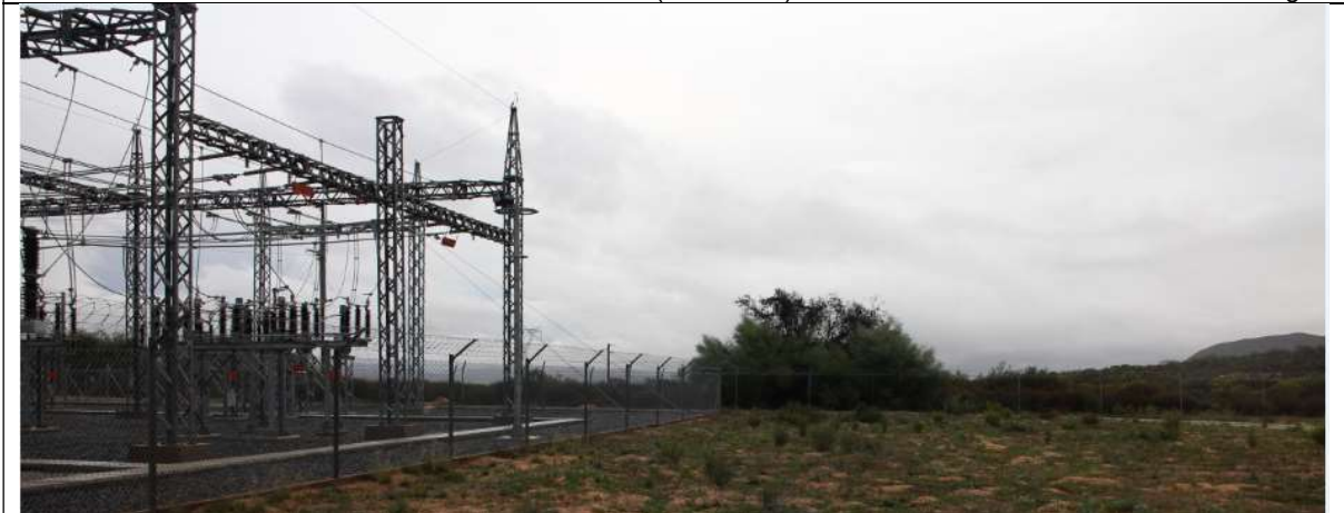
View of the area to the west of the Paleisheuvel Substation looking south
