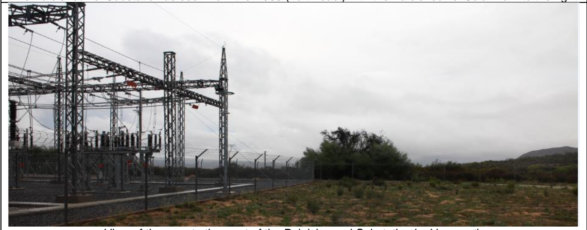
View of the area to the west of the Paleisheuwel Substation looking south
