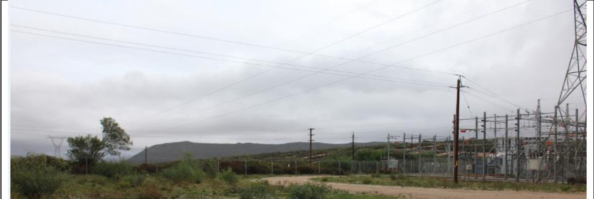
View of the Paleisheuwel Substation looking south
