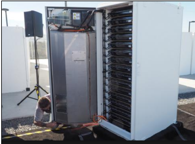
Figure 6: Solid state battery module
