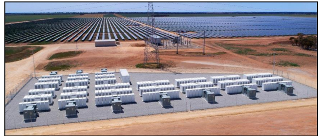
Figure 5: Example of a BESS
