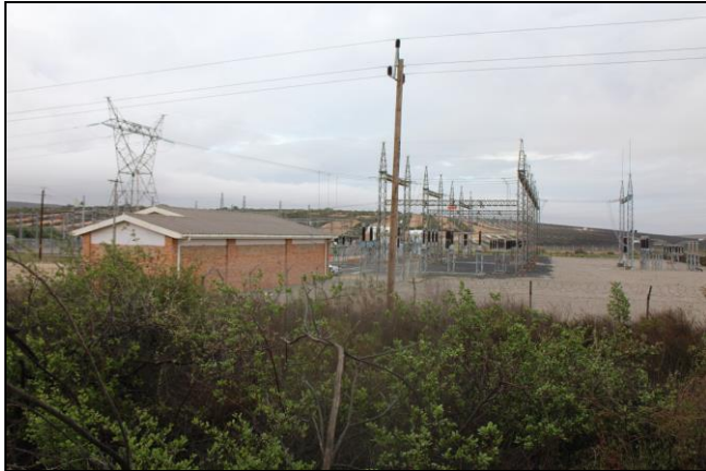
Figure 3: The Paleisheuwel Substation
