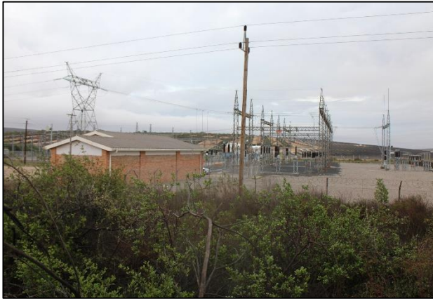
Photo 2-3: The Paleisheuvel substation
