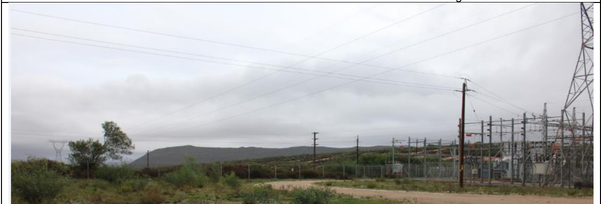
View of the Paleisheuvel Substation looking south
