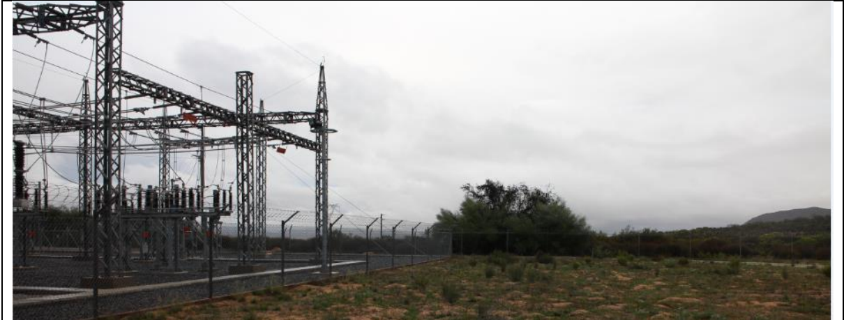
View of the area to the west of the Paleisheuvel Substation looking south
