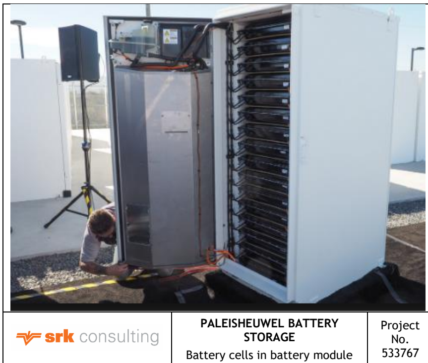
Figure 3-3: Battery cells in a battery module
