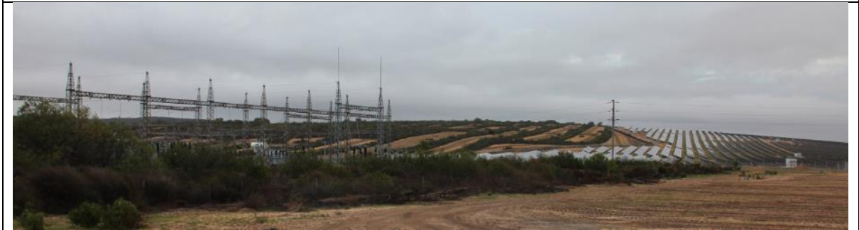
The Paleisheuwel Substation as seen from the R365 (north-east) with the Paleisheuwel Solar Park to the right
