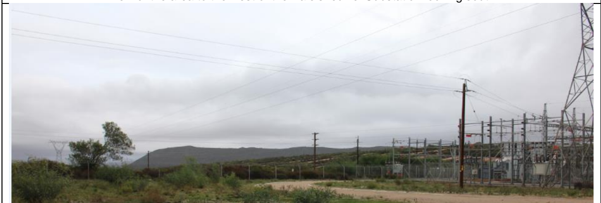
View of the Paleisheuwel Substation looking south
