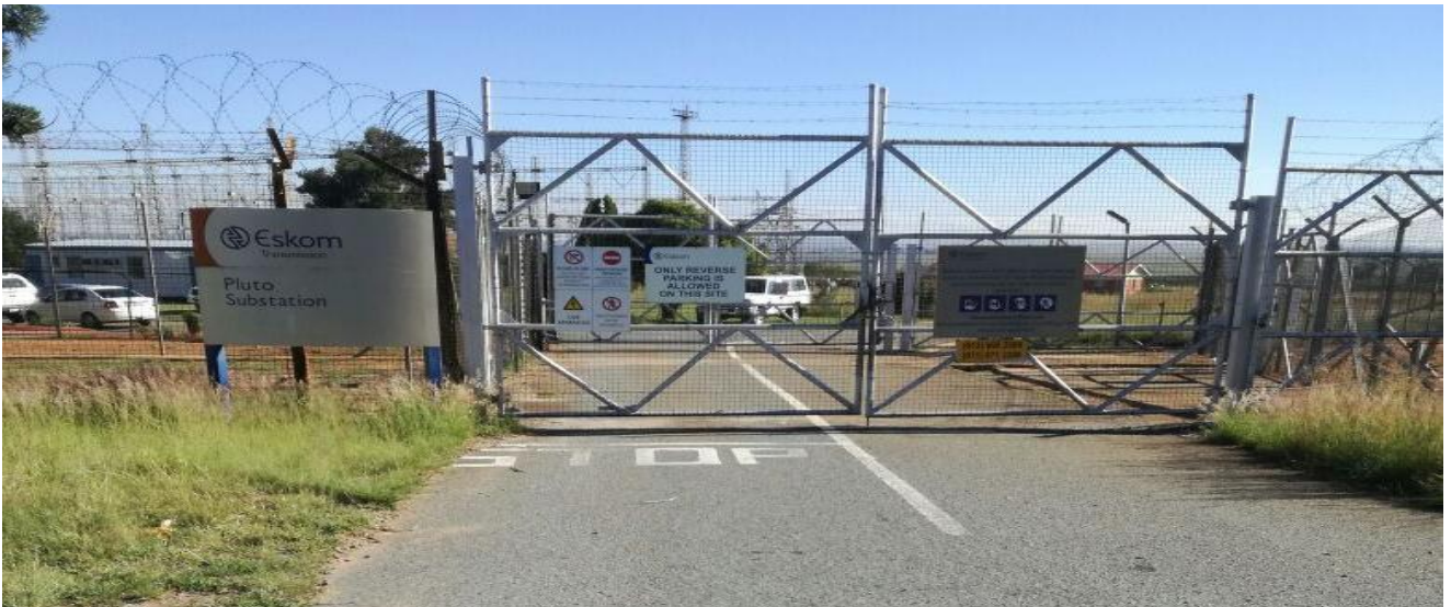
Figure 107: Pluto Substation in Gauteng
