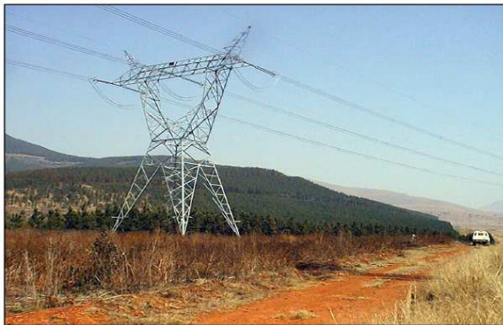
Self – supporting suspension tower
