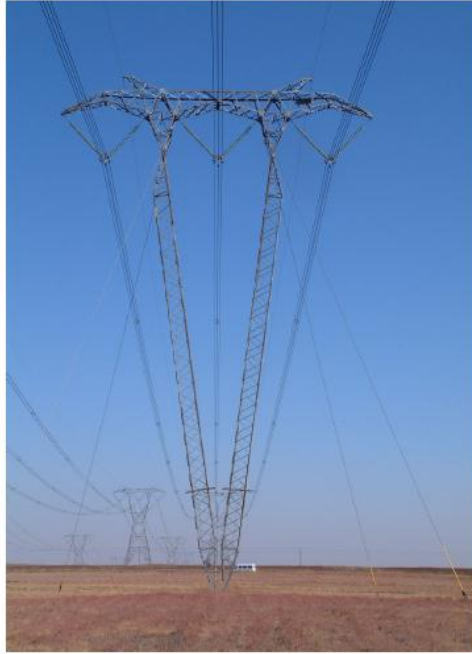
Figure A-5: Tower Type 520B (Guyed V).
