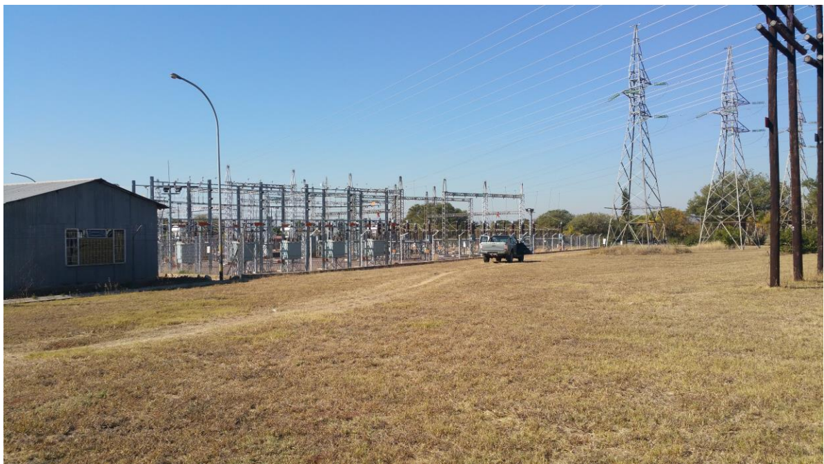
Photo i: the photo showing the Groblersdal Substation
