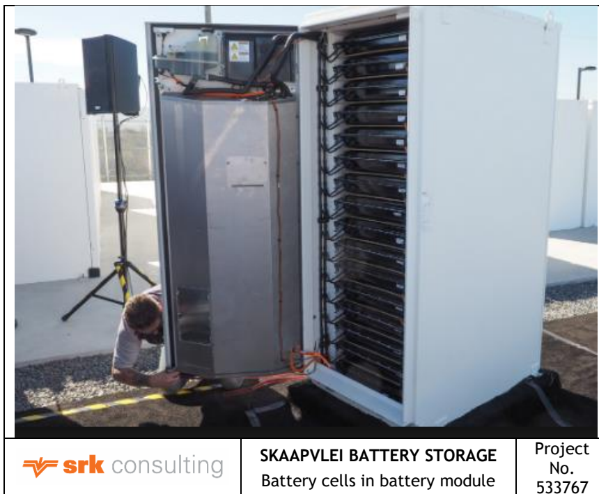
Figure 3-3: Battery cells in a battery module
