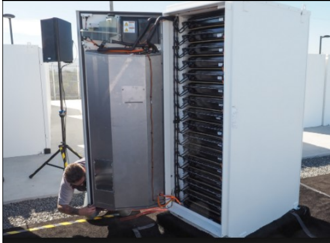
Figure 6: Solid state battery module
