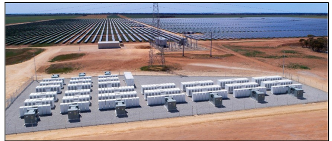
Figure 5: Example of a BESS
