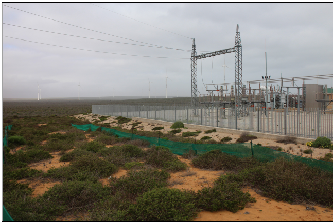
Figure 3: The Skaapvlei Substation
