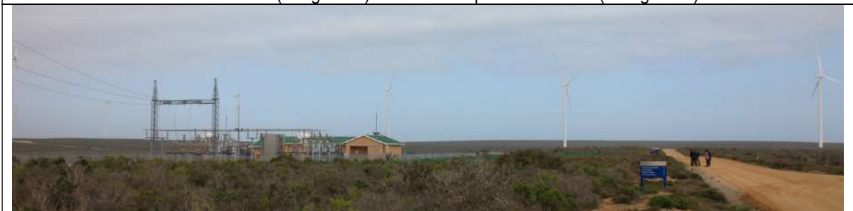
View of the Skaapvlei Substation from the access road looking west
