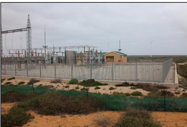
Photo 2-3: The Skaapvlei substation
