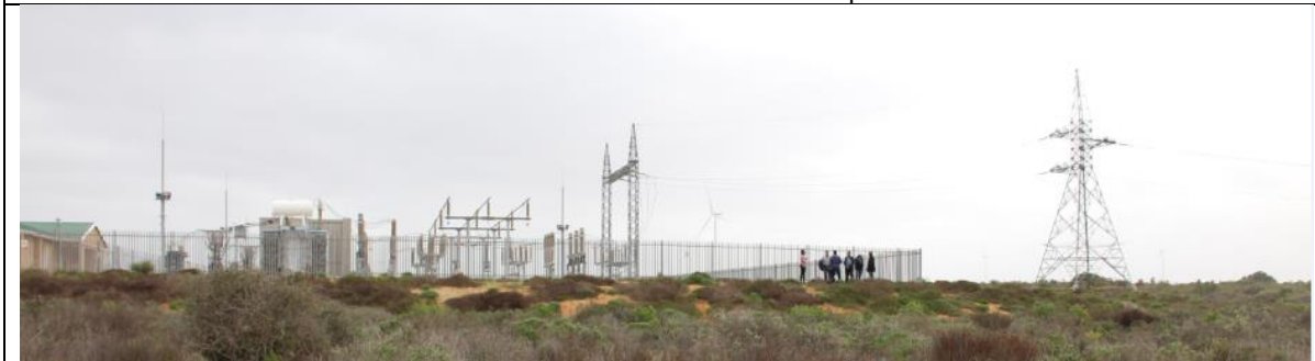
The Skaapvlei Substation as seen from the site
