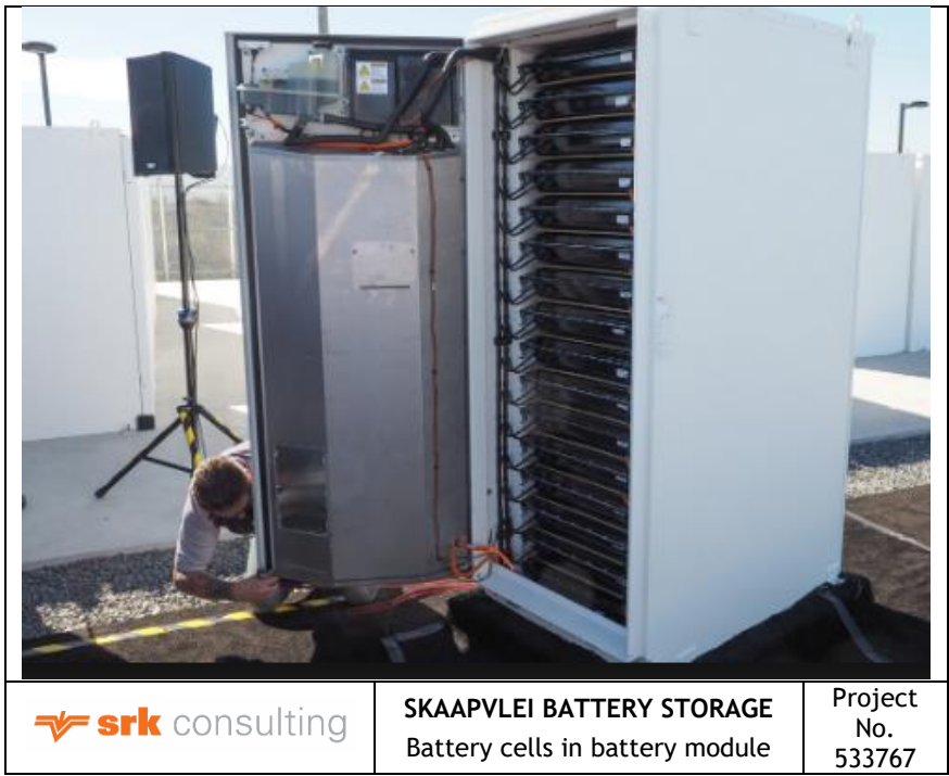
Figure 3-3: Battery cells in a battery module
