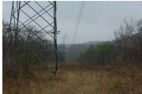
Figure 15: Undulating terrain and gorge to follow to Singo substation.
