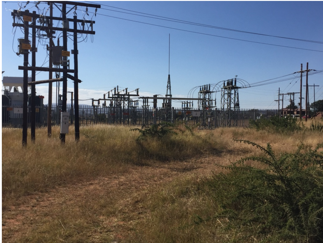
Photo 1: Existing Syferkuil Substation
