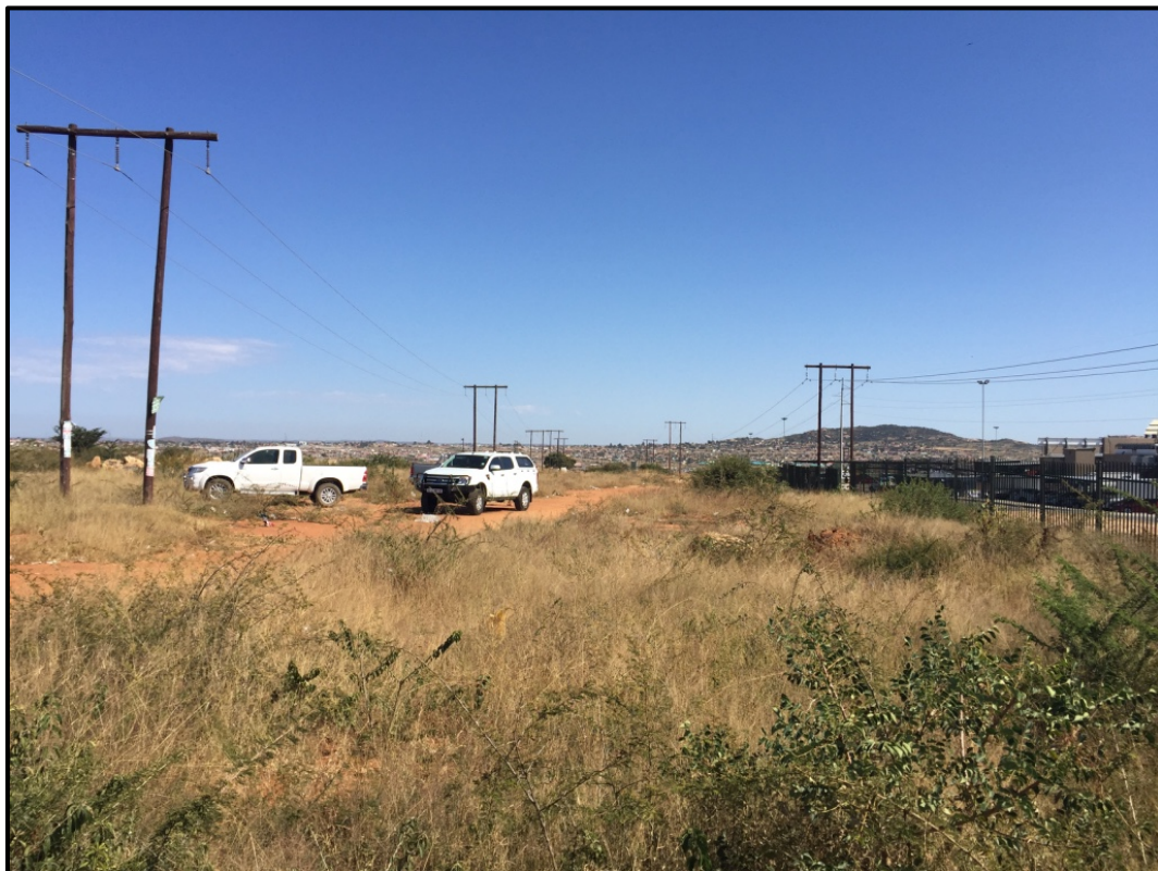
Photo 6: Thabampo-Syferkuil existing line on right and servitude near Thabampo Substation looking west
