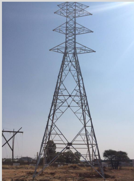
Photo plate 2: Steel lattice overhead structures
