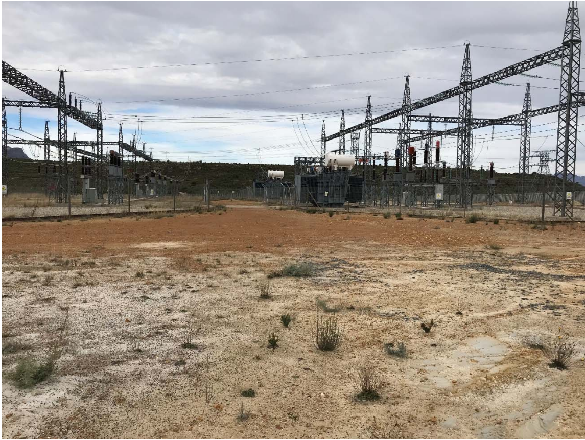
Figure 7: A view of existing infrastructure within the Witzenberg Substation
