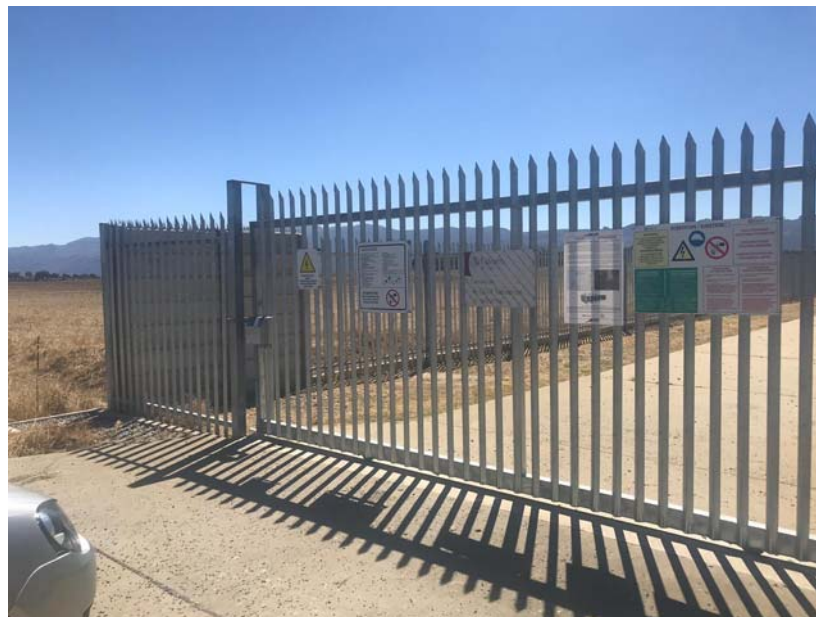
Figure 24: Notice board placed at the Substation gate
