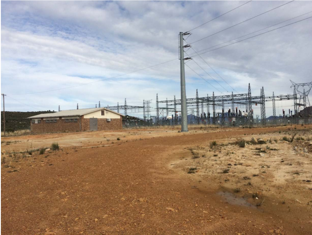
Figure 4: Highlights the orientation of the control house, switches, breakers within the Witzenberg Substation
