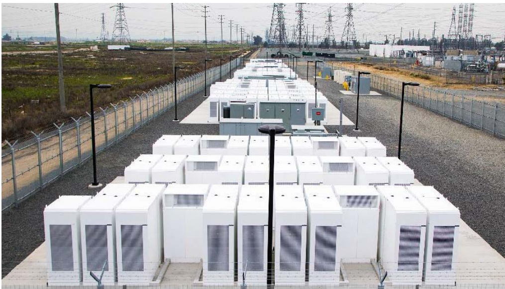
Figure 18: Lithium Ion BESS Facility
