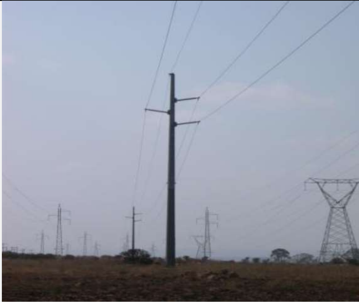
Figure 2: Single circuit steel mono-pole structures to be used for the Pylon structures
