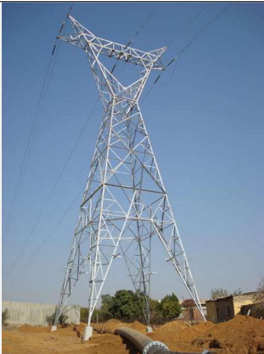
Figure 4: Single circuit steel lattice structure
