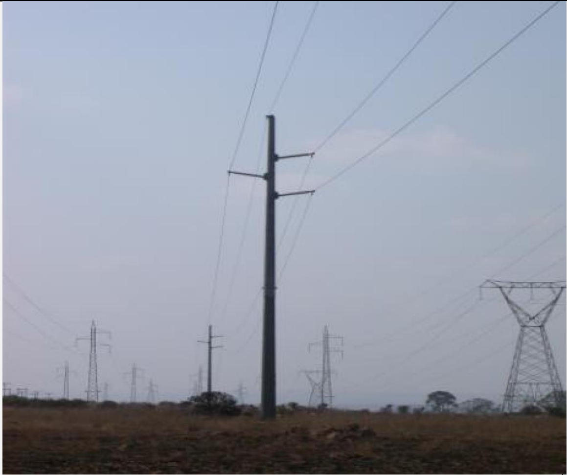
Figure 2: Single circuit steel mono-pole structures to be used for the Pylon structures
