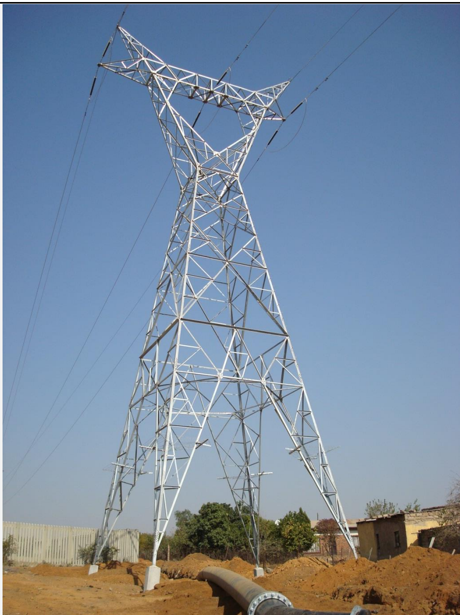
Figure 4: Single circuit steel lattice structures
