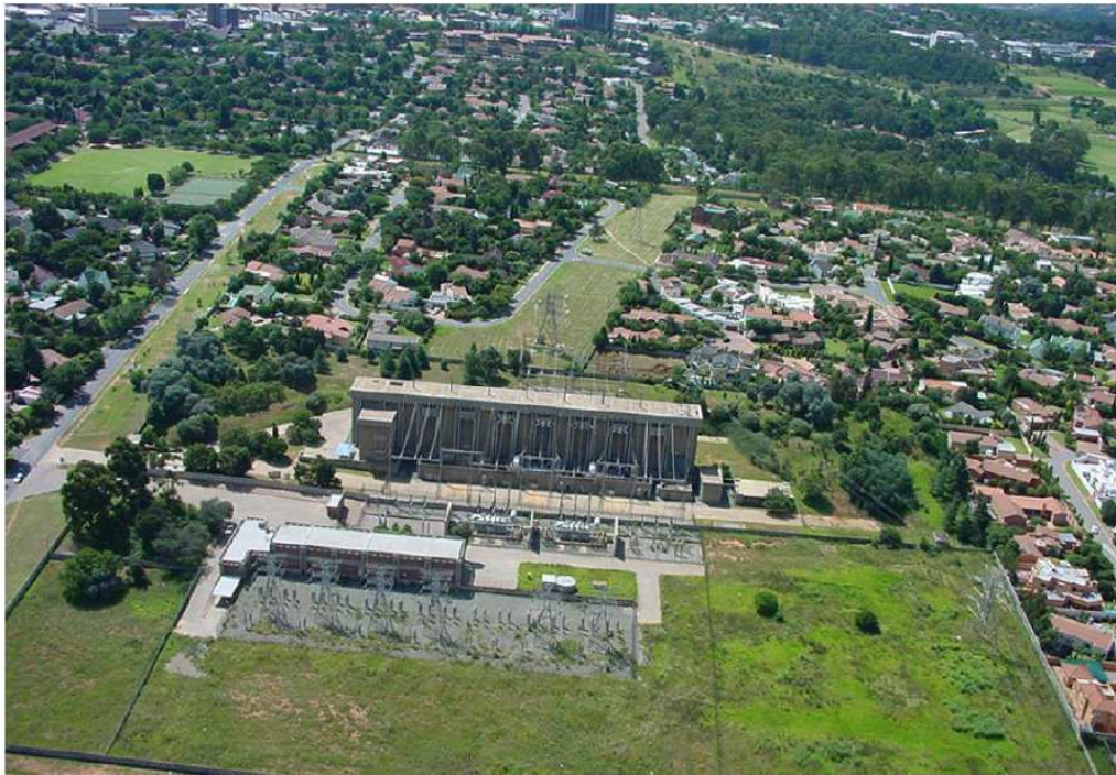
Figure 4-11: A typical Gas Insulator Substation
