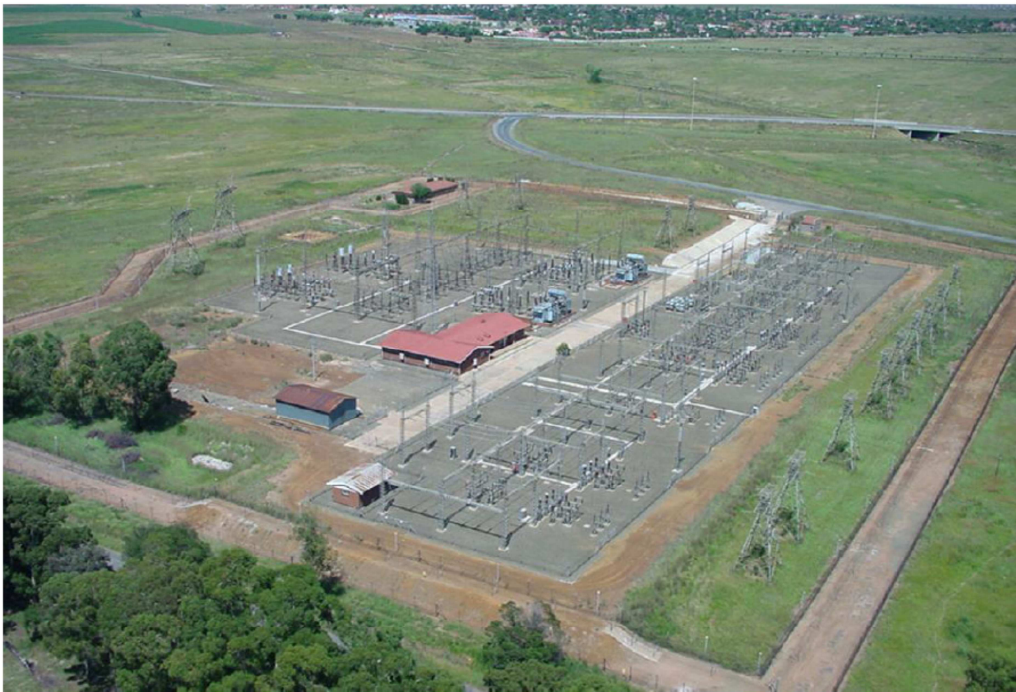
Figure 4-13: A typical Air Insulator Substation
