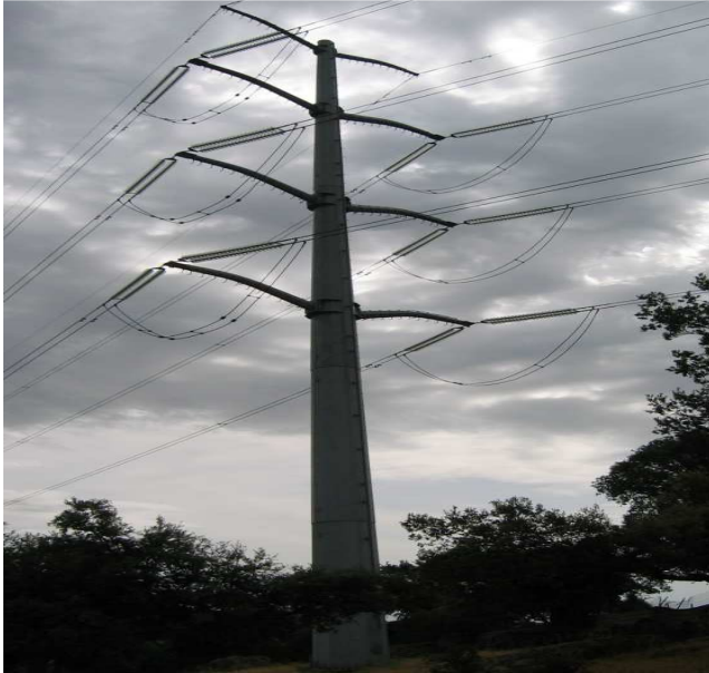
Figure 4-8: Steel Mono Pole
