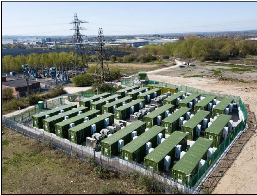
Figure 4: Example of a 29 MW BESS located in Aylesford, UK (Source: (Eskom, 2018))
